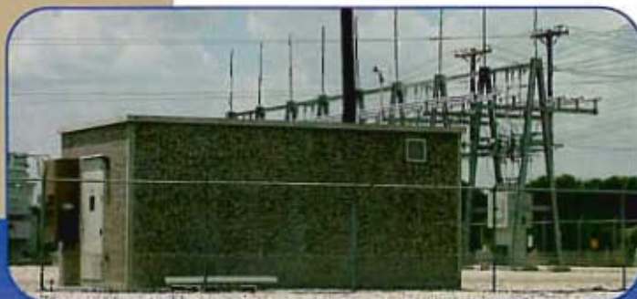
14' x 24' x 10' sub station control building.
