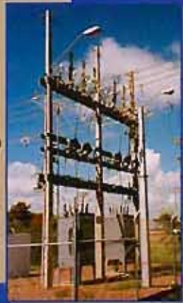
Substation area lighting and power distribution
